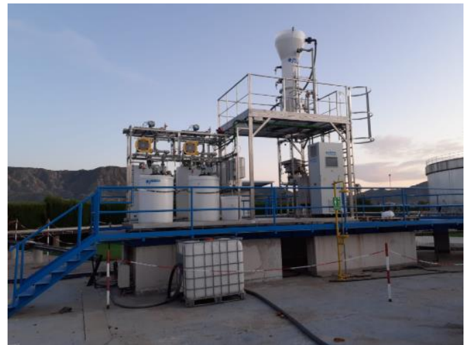
Struvite pilot plant
